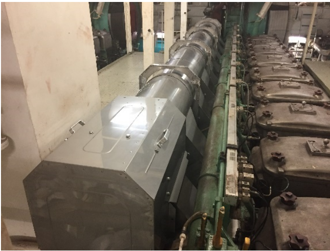
3. Turbocharger cladding, i.e. exhaust outlet and waste gate
